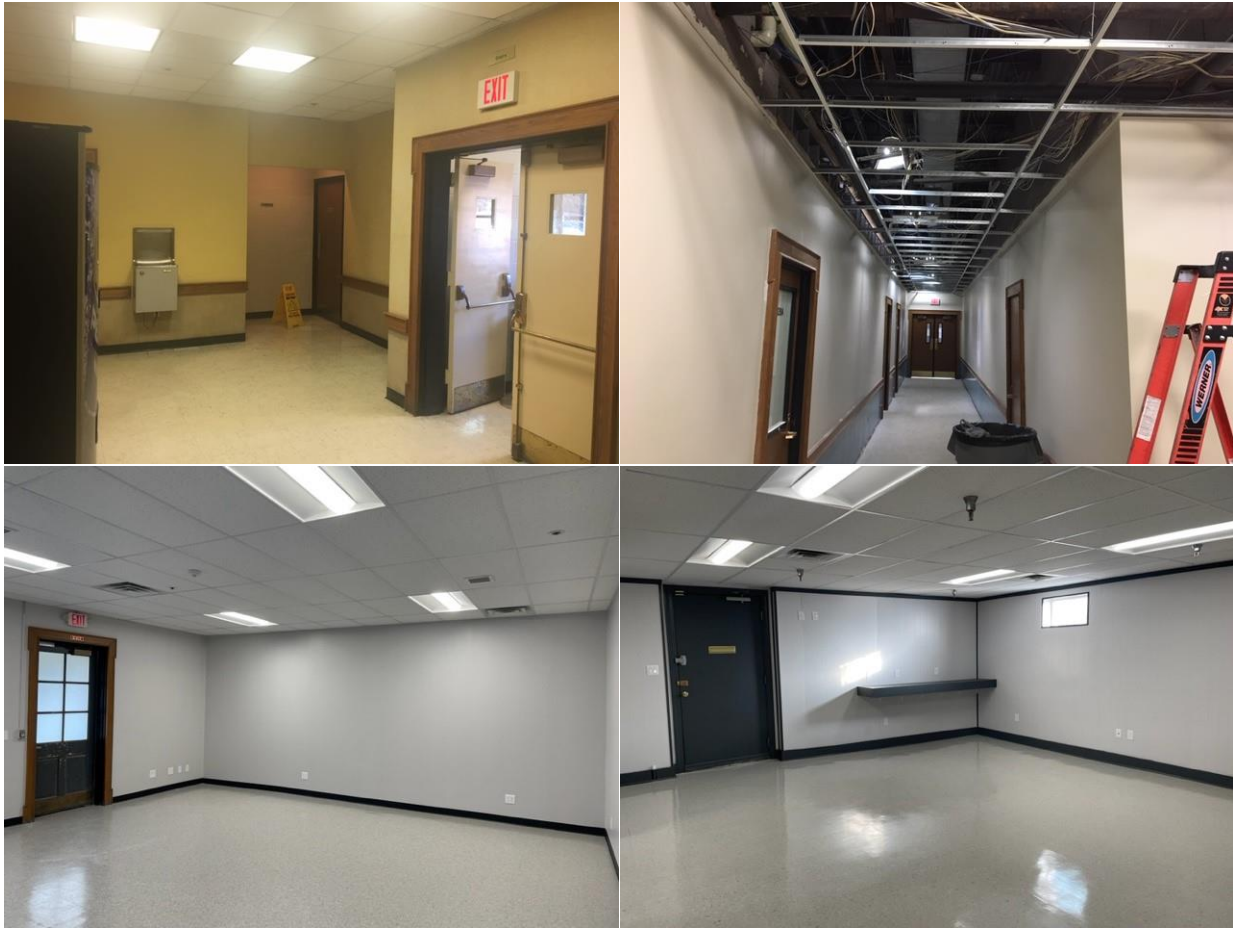
Figure 5: Images from before, during, and after LED lighting conversions performed by Facilities' Electricians at the Central Government Center and Electrical Maintenance buildings.
